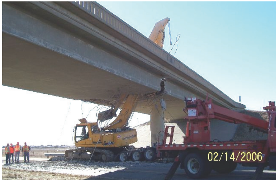
Figure 4.3.4 Accident Involving Construction Equipment and a Bridge
